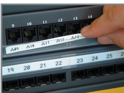
Punch Block & Patch Panel Labels
